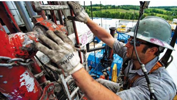
TOWANDA, PENNSYLVANIA Working 24 hours a day, crews in the Marcellus Shale drill for natural gas in this enormous play spanning the Appalachians from West Virginia through Pennsylvania.
