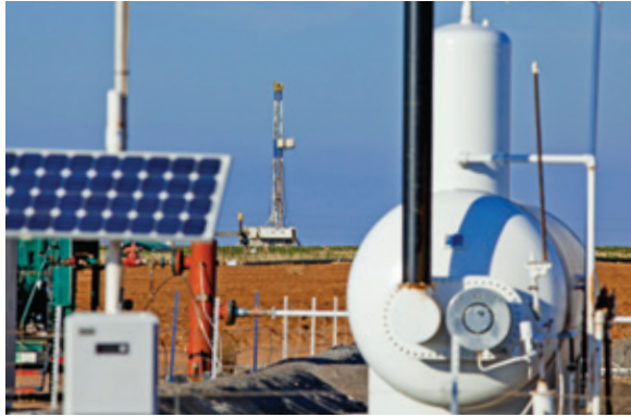
Solar technology is installed at production sites to power automation equipment.
