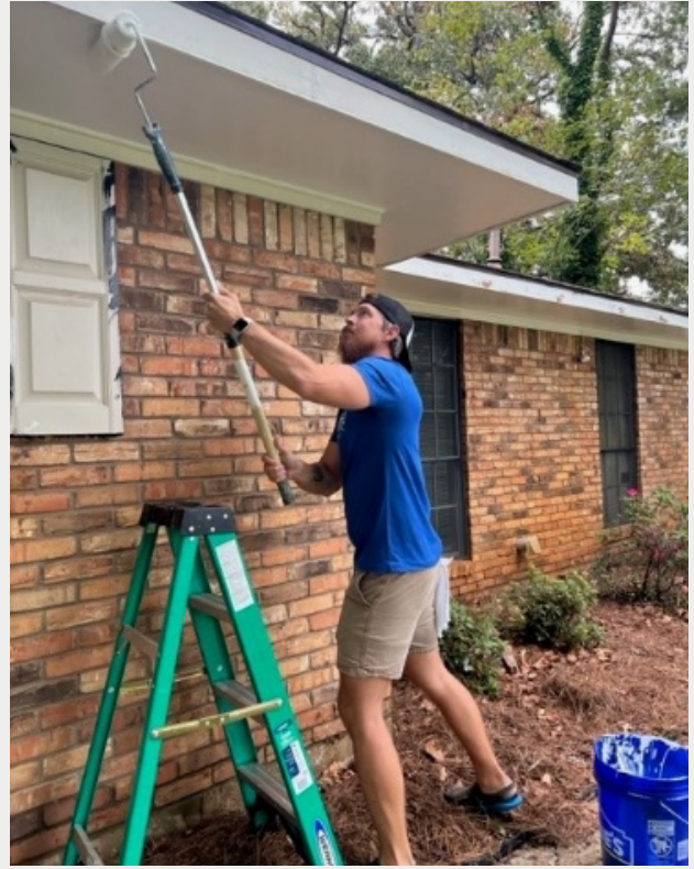
Cody Parker paints the exterior of the home during the volunteer project. The home will be used to house women and children in their program.
