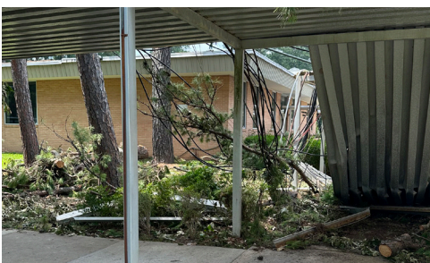
A severe storm carrying winds up to 80 miles per hour caused major damage and power outages across northwest Louisiana.
